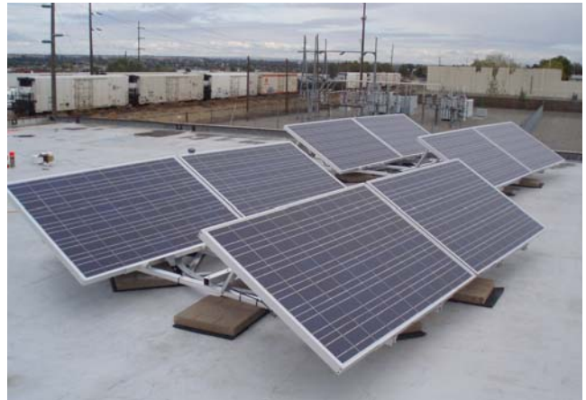
Figure 3: The two JXC SunTrack Carousels shown here were installed in Eastern WA in October of 2007.
