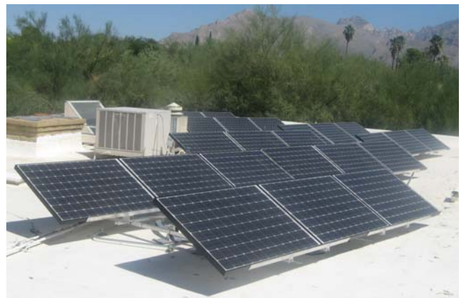
Figure 4: Four JXC SunTrack Carousels on rooftop in Tucson AZ (4.68 kW). Six Sanyo modules are mounted on each carousel in 2 rows with 3 modules per row.
